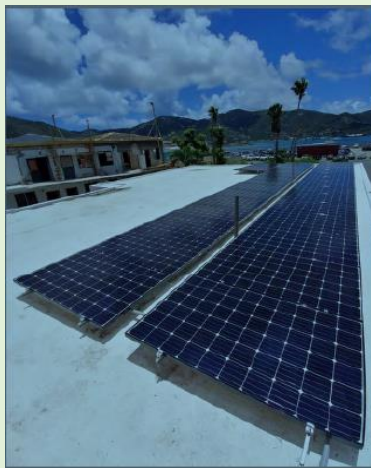
B: Solar panels on roof
